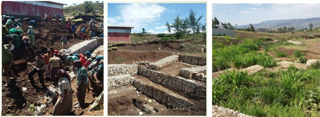
Figure 5 Gully Reclamation at Haromingna Kebele
